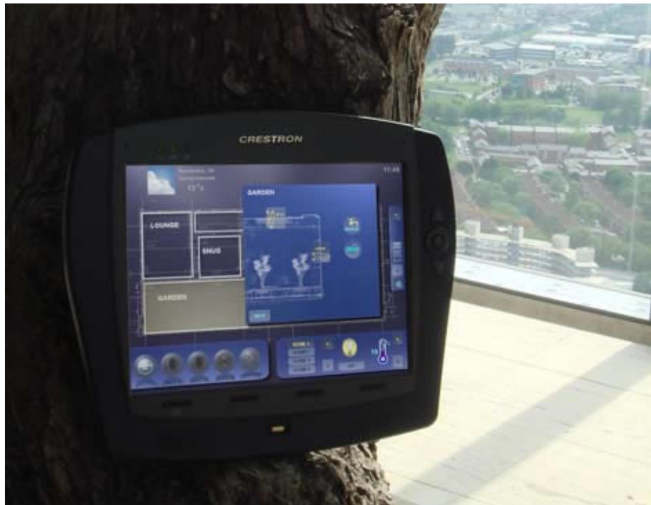
Crestron touchpanel being used for controlling HVAC and lighting in the Penthouse of the Beetham Tower, Manchester.
